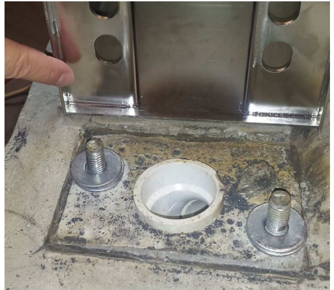
Install three to four washers on each anchor to fill the gap between the concrete and the tower.
